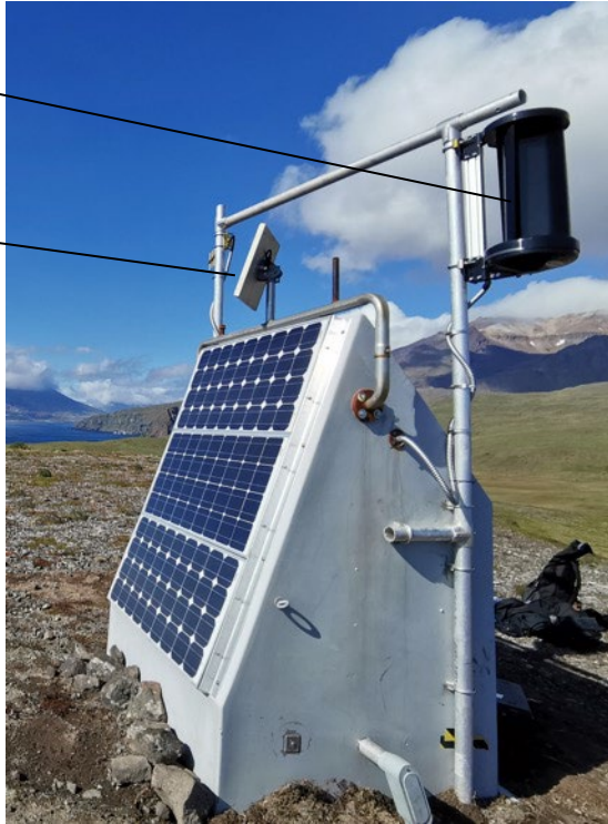
CLCO Comms Hub on Cleveland Sept 2022
