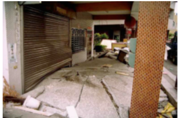
Figure 2. Typical foundation failure (punched footings and intermediate slab heaving). Chu et al. 2008. Photo by R. Seed (1999).
