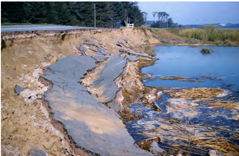
Figure 14. Ground failures in highway fill along the margin of Lake Merced along Lake Merced Blvd from the March 22, 1957 earthquake. (Photograph by M.G. Bonilla of the U.S. Geological Survey).
