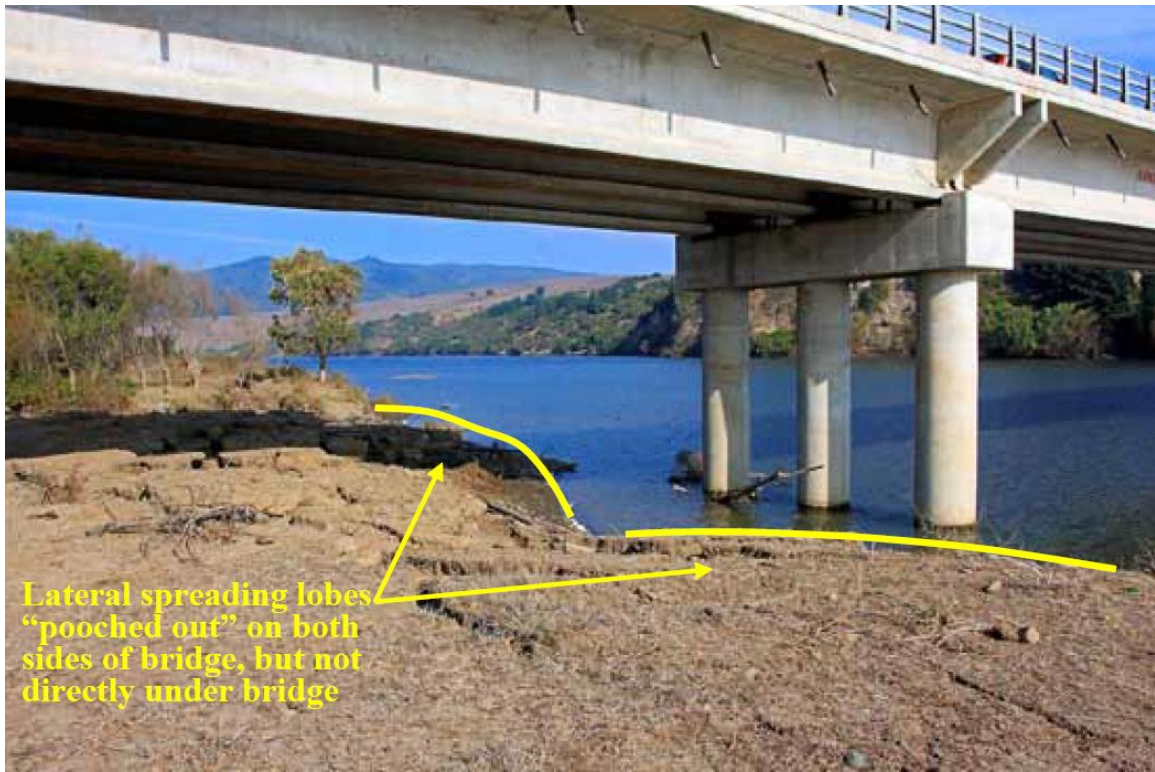
Figure 3.21: Lateral spreading at the northeast abutment of the Mataquito Bridge (From FHWA, 2011).
