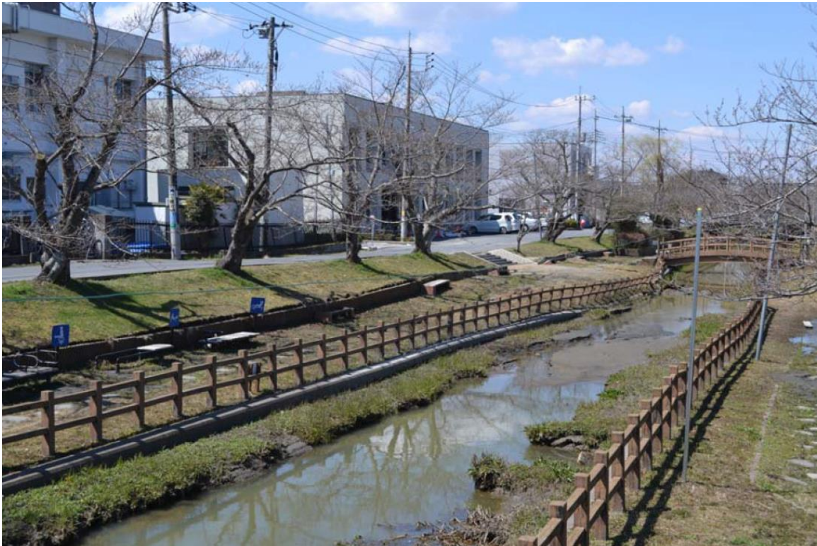
Figure 3.4: Displacement of channel banks in Katori due to lateral spreading (Ashford et al. 2011).
