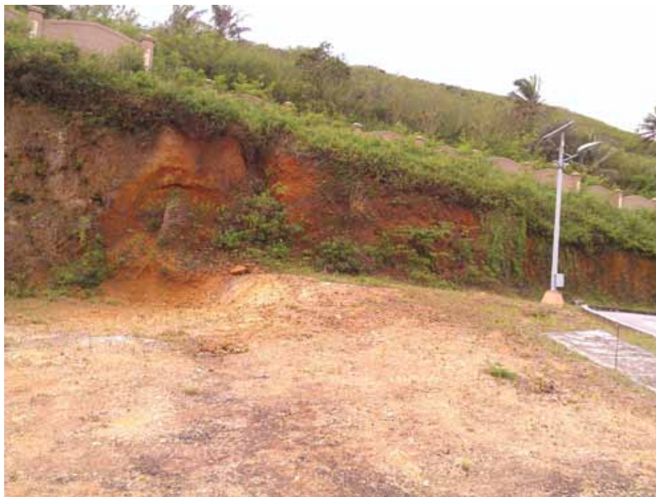
Bedrock fault extending across homesites into scarp. View to the west.
